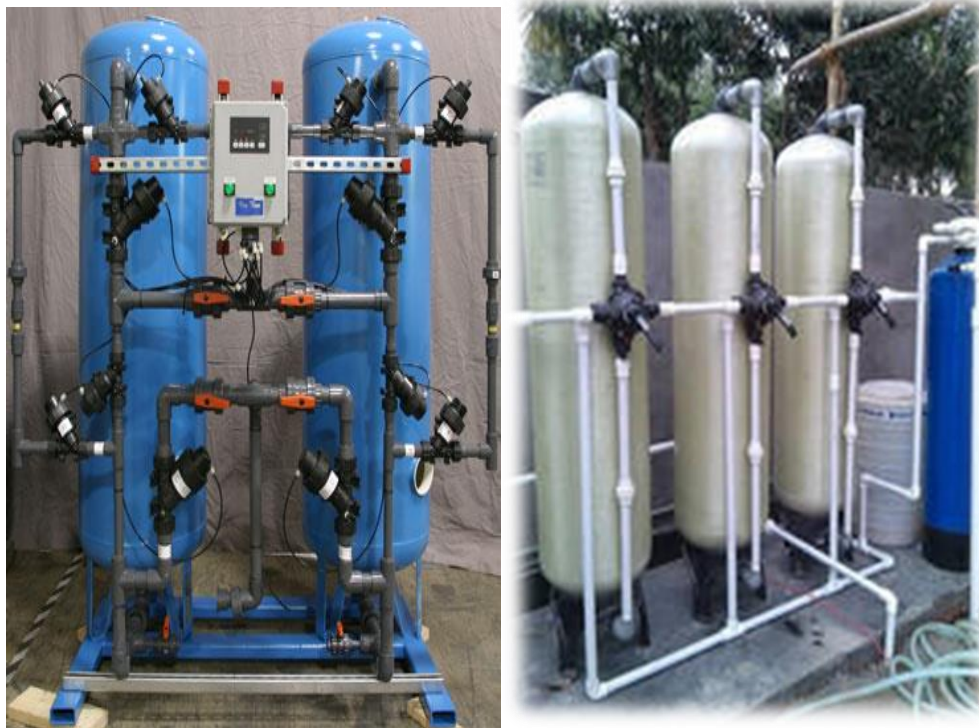
Fig: Water Treatment Plant
